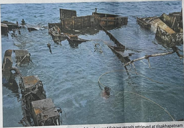
Debris clean-up: Workers cutting the parts of the drowned fishing vessels retrieved at Visakhapatnam Fishing Harbour on Monday. K.R. DEEPAK
