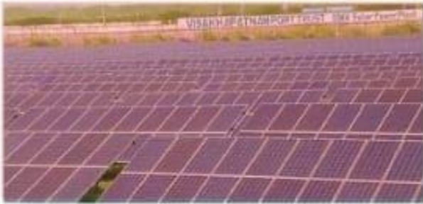
A view of the solar power plant at Visakhapatnam Port Authority
