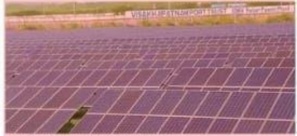
A view of the solar power plant at Visakhapatnam Port Authority
